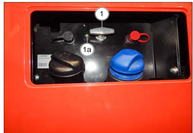
Figure 66: Battery disconnect switch
