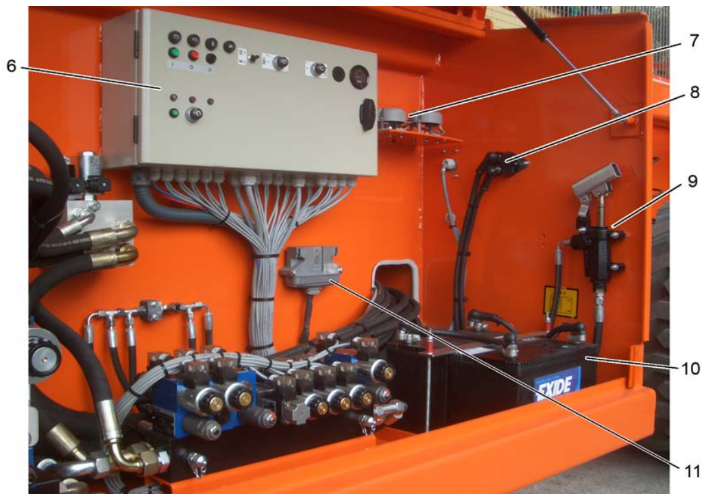
Valves and generator
