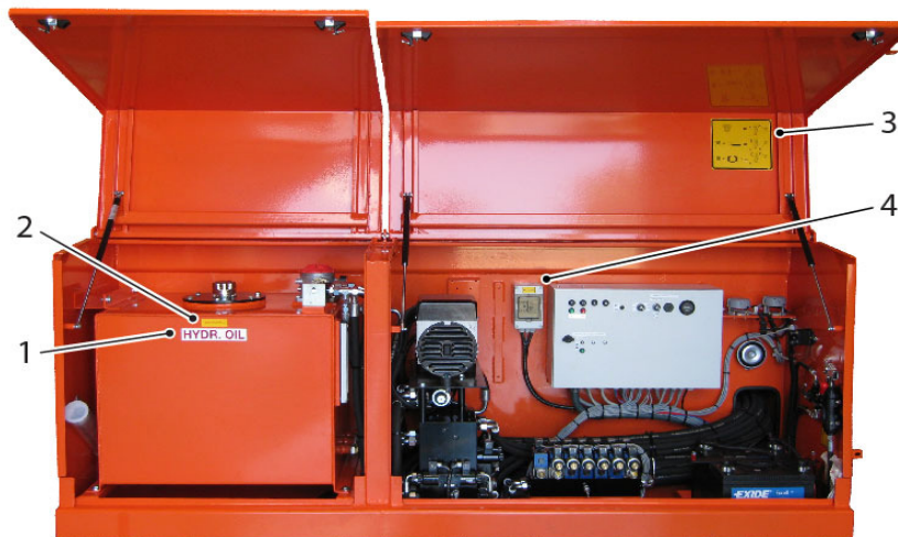
Hydraulic oil and valve/electrical compartment
