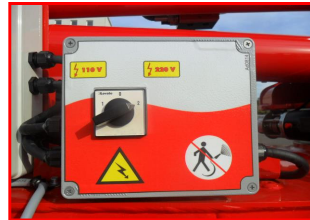
Picture 8b: transformer box with voltage selector.
